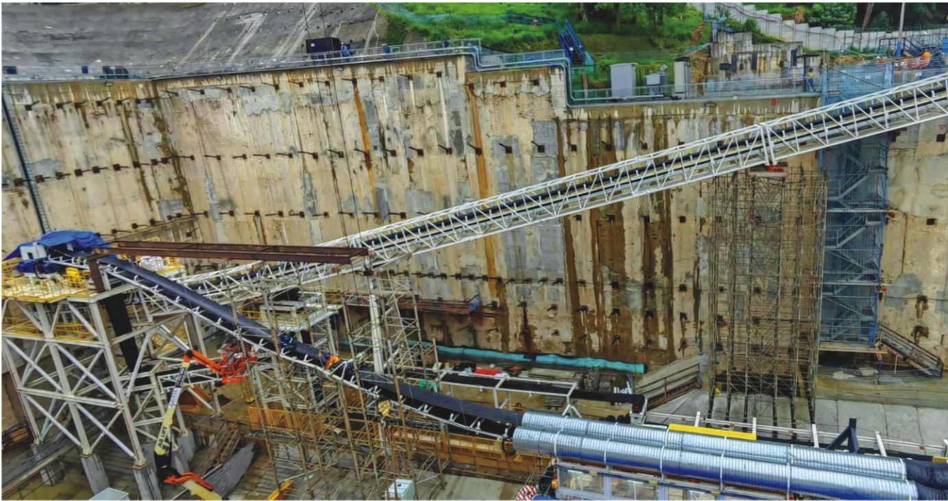
The large inclined transfer belt conveyor realizes the initial slag discharge of TBM.
