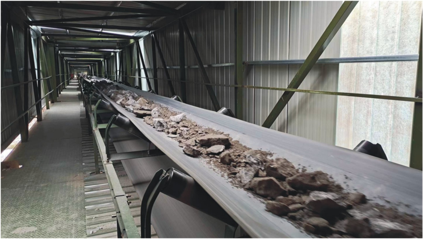
The enclosed corridor belt conveyor achieves safe, eco-friendly and dust-free transportation.
